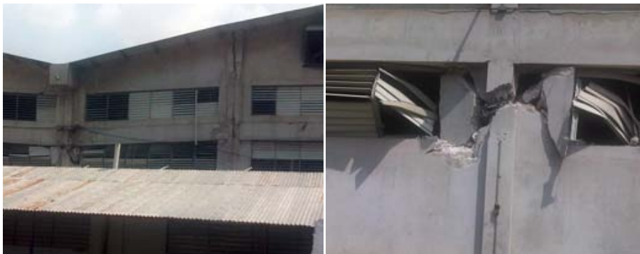
Structural damage to Haiti building Closer view of damage
